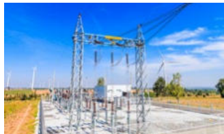
Substation partial discharge
